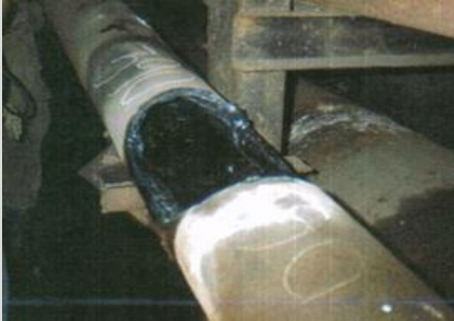
Inspection hole directly after the pump
