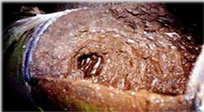
Contaminated pipe in 90% cross-section
